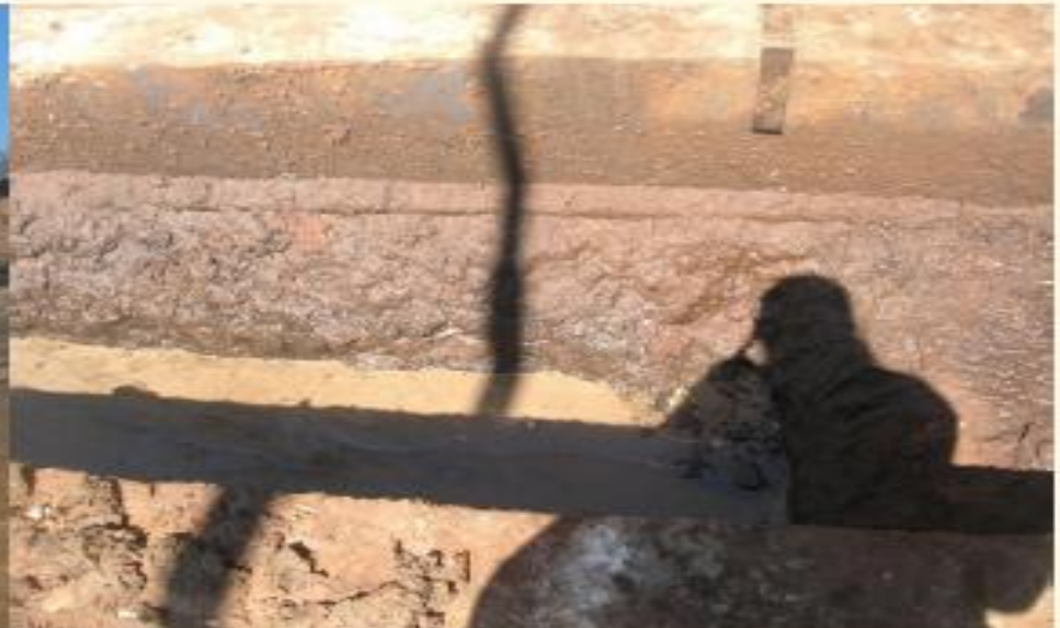
Oil Contaminated silts in the drainage from wash bay -Chibuluma Mining Plc
